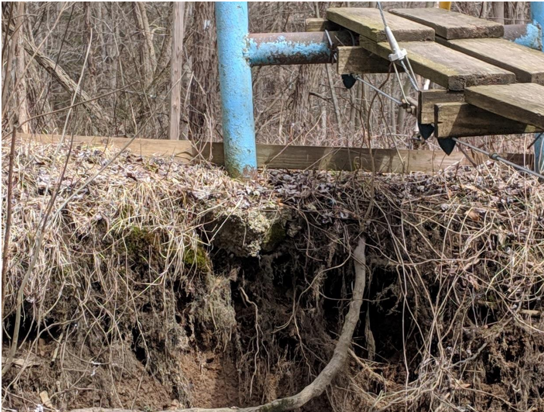
Figure 2: Close-up of the eroded bank under the suspension bridge footing.
