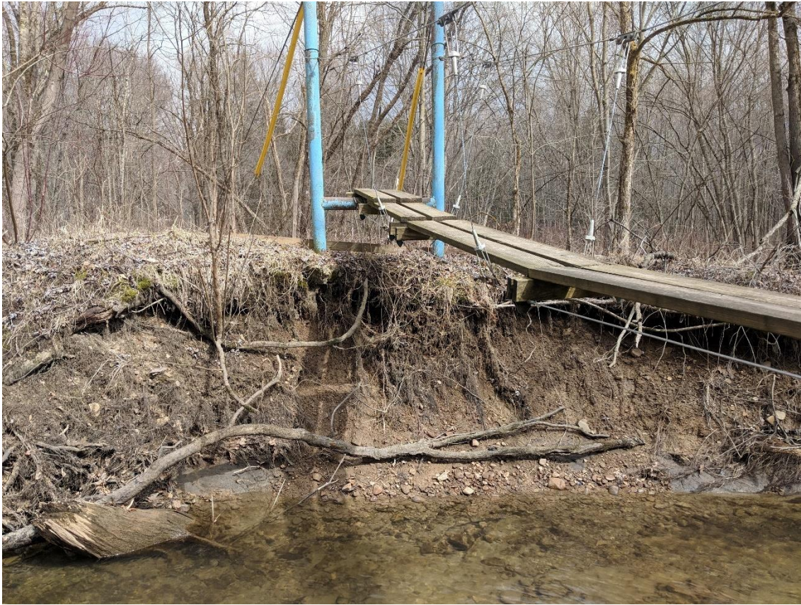
Figure 1: The banks of the stream are eroding away the base of the existing suspension bridge.
